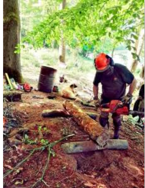
De-barking logs prior to charring to dry them out for use as load bearing columns
